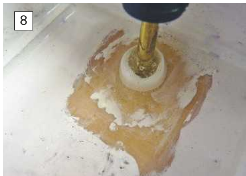
PHOTO 8. The rudder post tube is supported by a 'block' of epoxy adhesive within a small surrounding piece of plastic plumbing tube.
