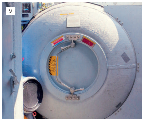
Photo 9. The entry hatch of the decompression chamber, seen here from the port side and looking forward to starboard.
