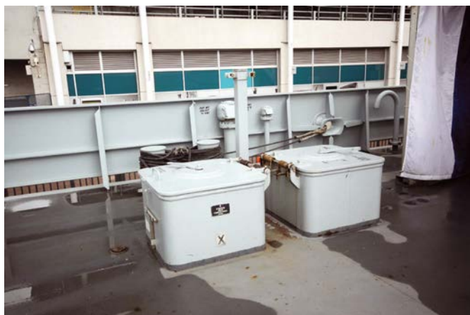
Cargo deck fittings
