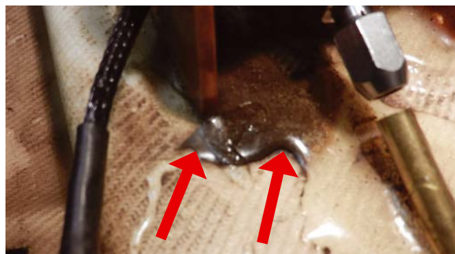
Arrows show the areas where the water is coming into the hull (see text)
