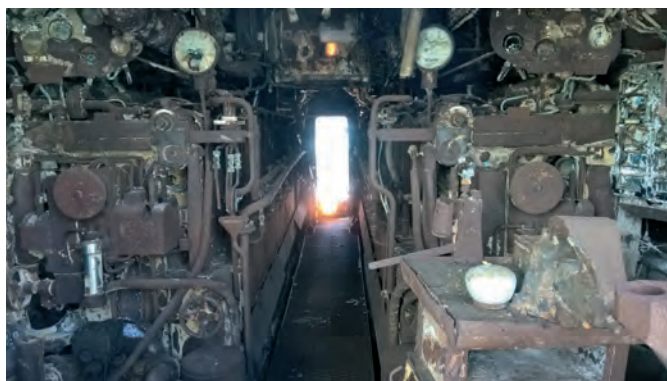
The Diesel motor room
