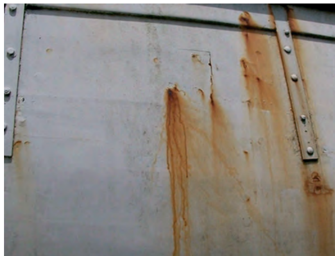
It's not only steel hulls that rust. Rust leaching through a wooden hull
