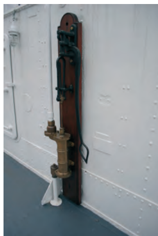
The pump is an original feature
