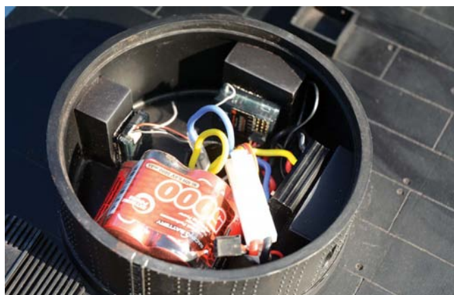
The electrics are quite a snug fit inside the turret but at least they're dry
