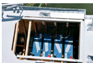
The four 6 V/10 Ahr batteries installed under the bridge. You can see the lead ballast in the front
