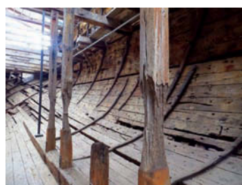
The deck supports eaten away between high and low water mark
