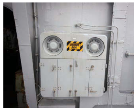
Comms box starboard side
