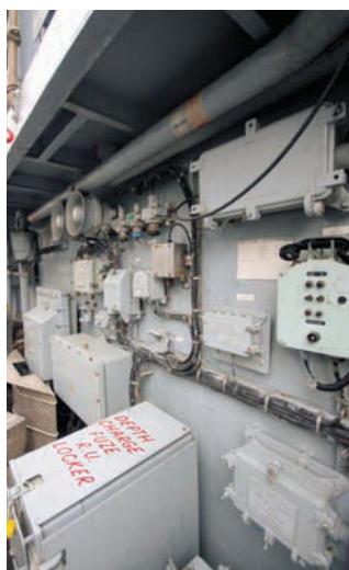
Details of dials and switches on forward end of rear superstructure
