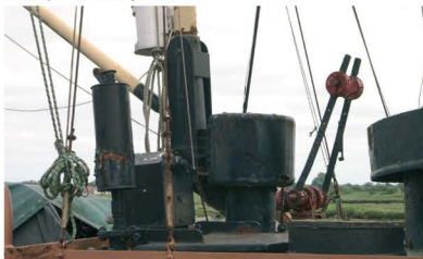
Engine room exhaust and air intakes
