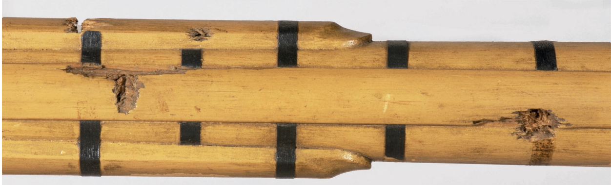
Detail at the lower end of the cheeks showing gouges and impact scars from cannon fire damaging the cheeks and front fish.
