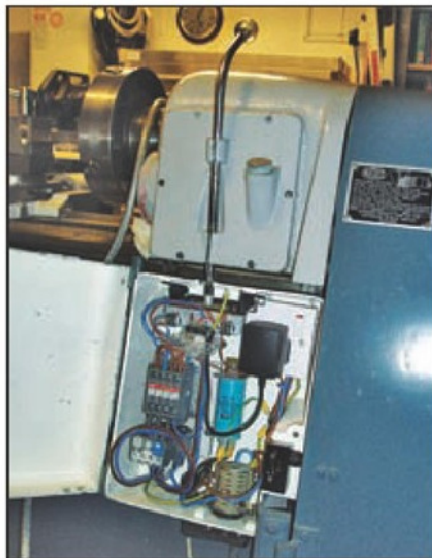
12. The electrical controls.
