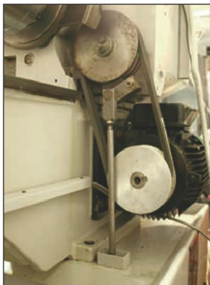
3. The original drive arrangement.
