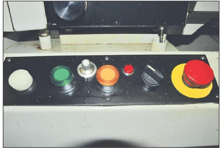
Photo 6. The switch box.
