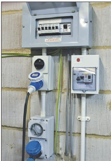
Photo 7. Properly installed electrics.
