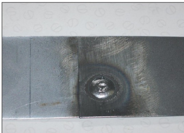
Photo 9. Top side of fake 'spot' weld.
