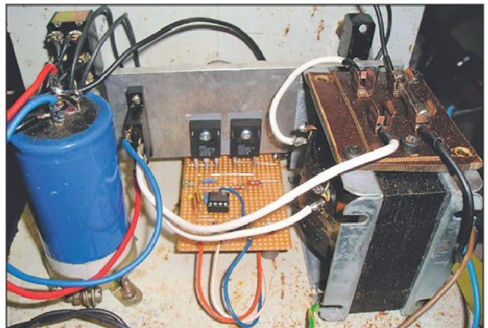
Photo 16. Inside of the controller.
