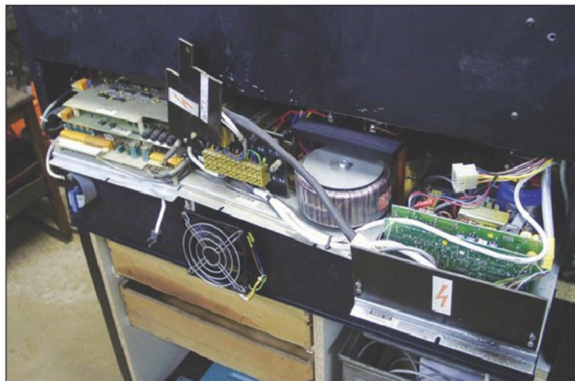
Photo 2. Chassis partly drawn out to rear showing electrical sub assemblies. Left to right, Board stack, Power supply unit, Spindle variable speed drive.
