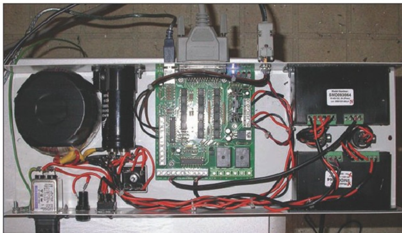
Photo 2. The electronic control box.
