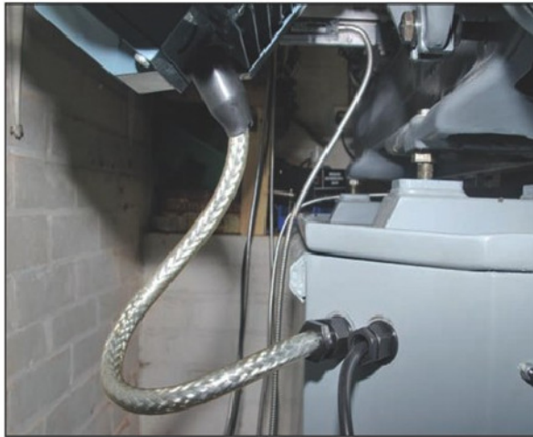
Photo 14. Motor and Mains cable Glands.
