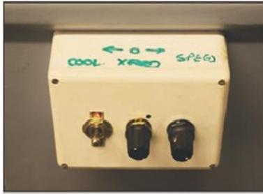
Photo 21. Coolant and power cross feed control panel.
