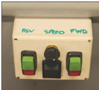
Photo 16. Lathe and inverter control panel.
