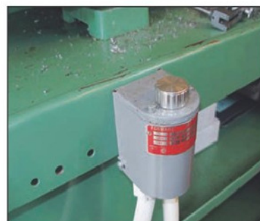
Photo 15. The lever on the switch has been replaced by a round knob.
