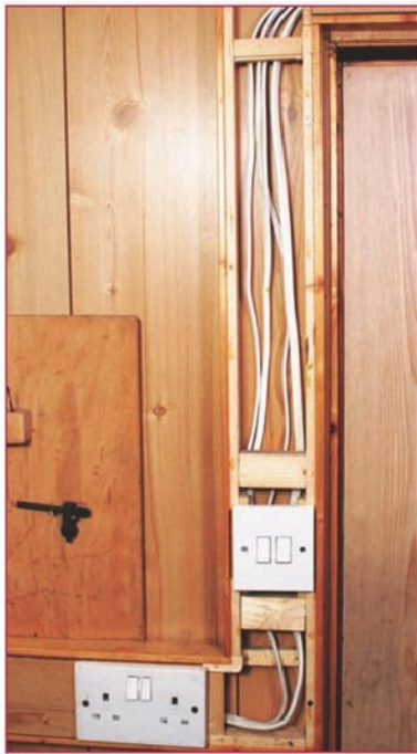
9 A method of installing the electrics that is tidy, easy to install and easy to modify.
