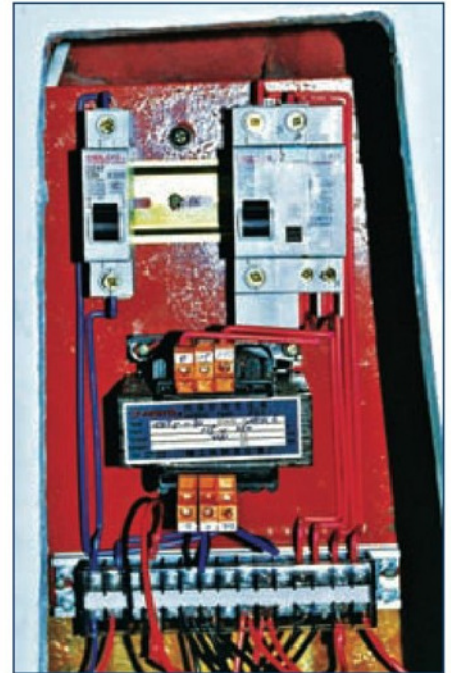
4. Mill electrics inside column.
