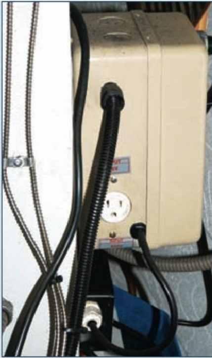
2. "Align" step down transformer on back of column.
