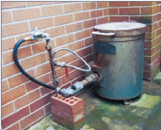
1. Furnace connected to gas supply.
