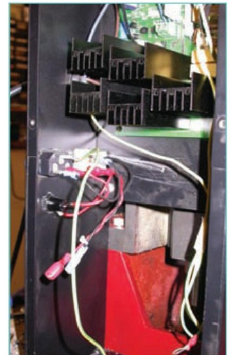
10. Interior of housing awaits transformer.
