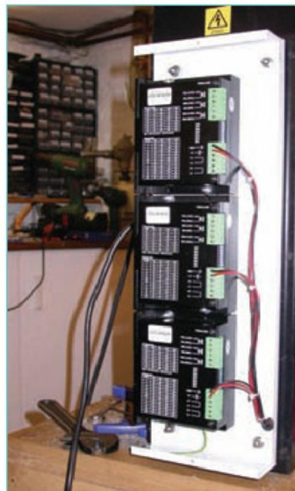
12. Controller mounting box fitted with three stepper drives.
