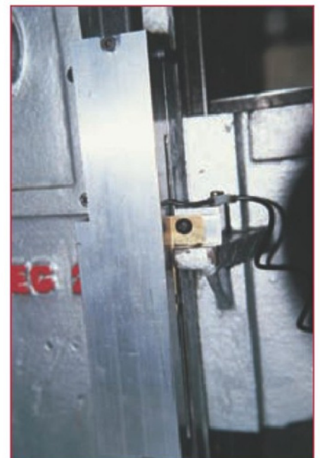
14. Protective cover fitted to the scale shown in Photo 13
