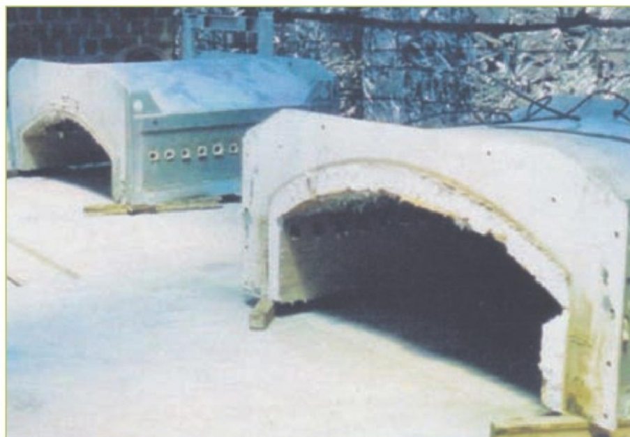
8. The two part roof and integral electric heating system were completely blown off the furnace by the force of the steam explosion.
