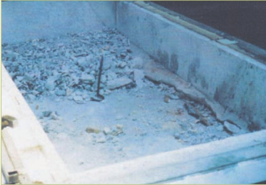
7. The furnace hearth following the explosion caused by using excess water in the mix.
