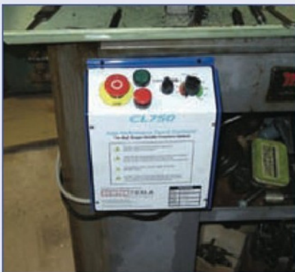
2. Inverter control box located in place of "Dupar" reversing switch.
