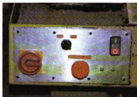
3. The new control panel which allows 'Remote' operation
