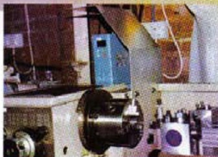
1. The Eurotherm drive is mounted behind the headstock. The aluminium shield allows adequate ventilation whilst guarding against the ingress of swarf
