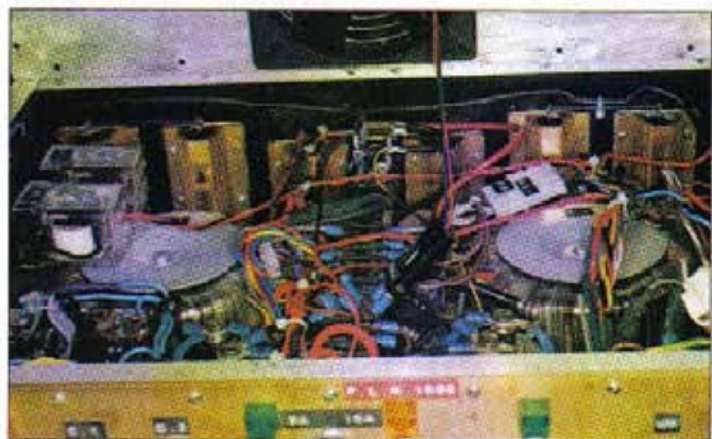
22. Inside showing the relays to the left
