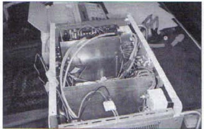
39. A further view of the compartmentalised control cabinet
