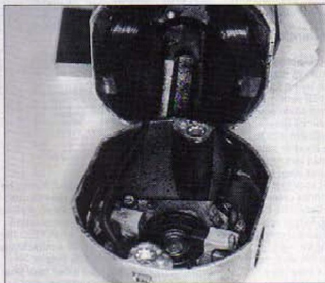
1. The end cap and brush housing of the motor before cleaning.
