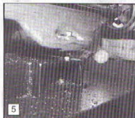
5: Position of the drip tray drain pipe.
