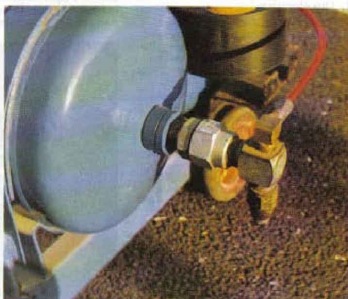
The inlet end of the reservoir showing the plastic feed pipe from the compressor, and the one way valve on the reservoir.
