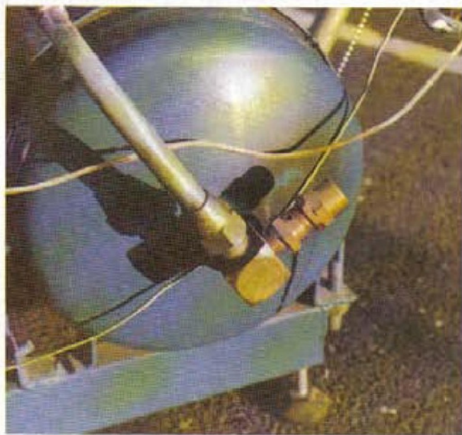
The outlet end of the reservoir, showing the brass safety valve.
