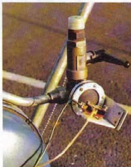
A close-up of the pressure switch. This is a home made unit designed to switch at low pressures, not exceeding 30 p.s.i. The tap seen above it is not part of the switch!
