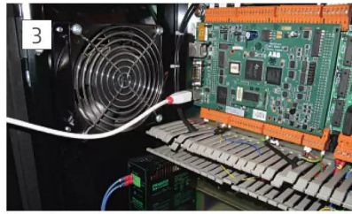
The control card with the direct cable from the laptop connected.
