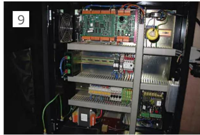
The control cabinet
