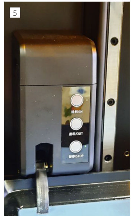
The 'smart pump' has manual controls as well as automatic functions.
