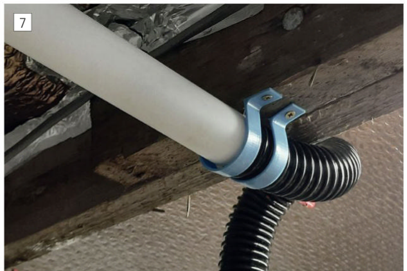
A section of my 'ventilation system'.
