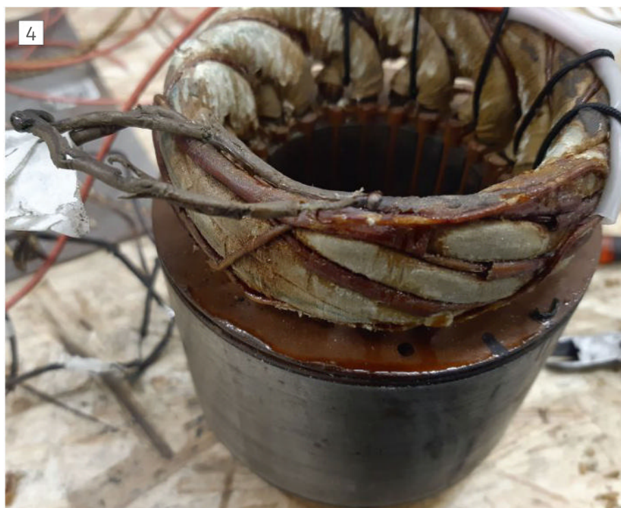
Detailed picture of damaged leads. Just visible at the top right is the routing of the first new wires and silicone-rubber insulating tubes.
