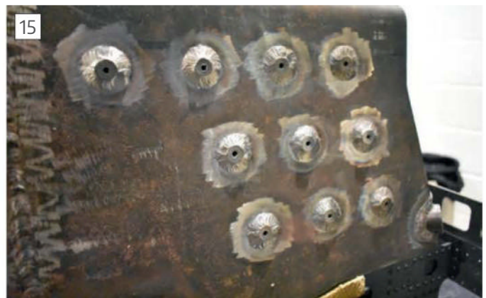
Steel boiler with tell tale holes in the firebox stays.
