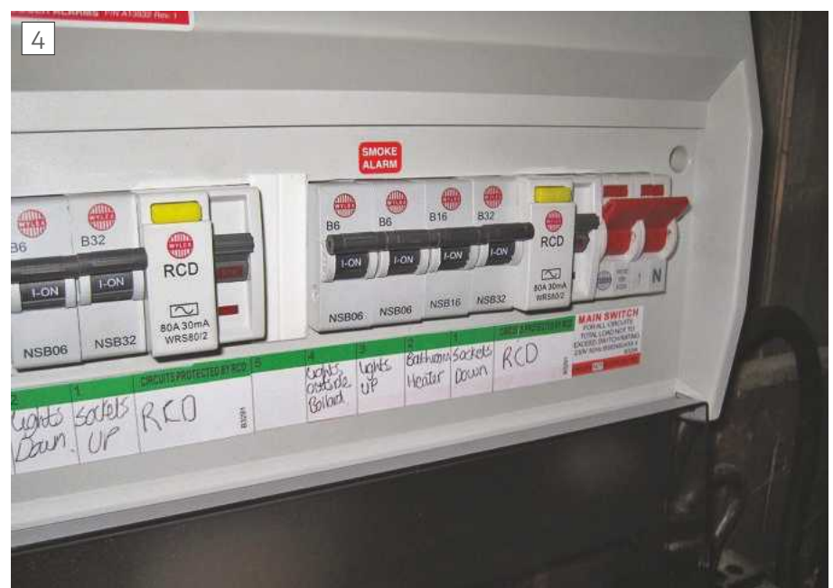
Distribution board with MCBs.
