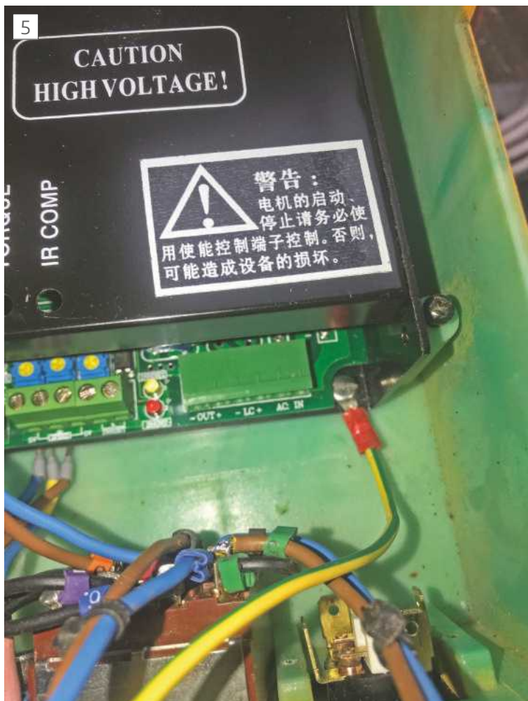
Controller Earth Connection
