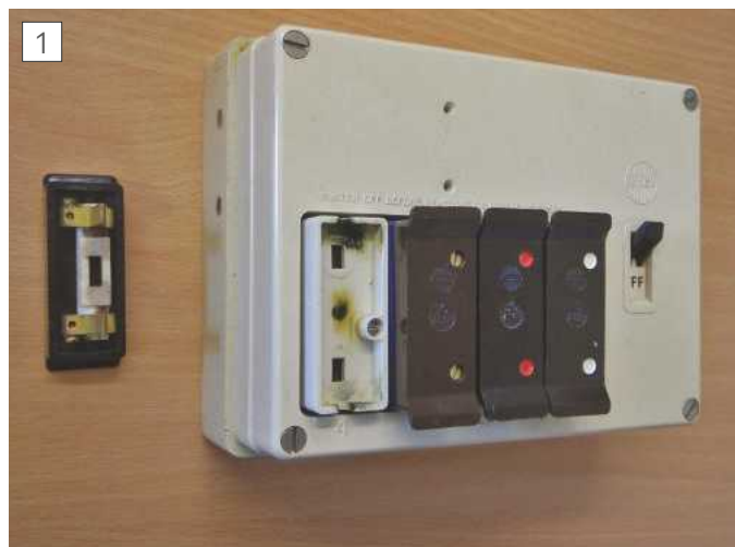
Old style distribution box with rewireable fuses.
