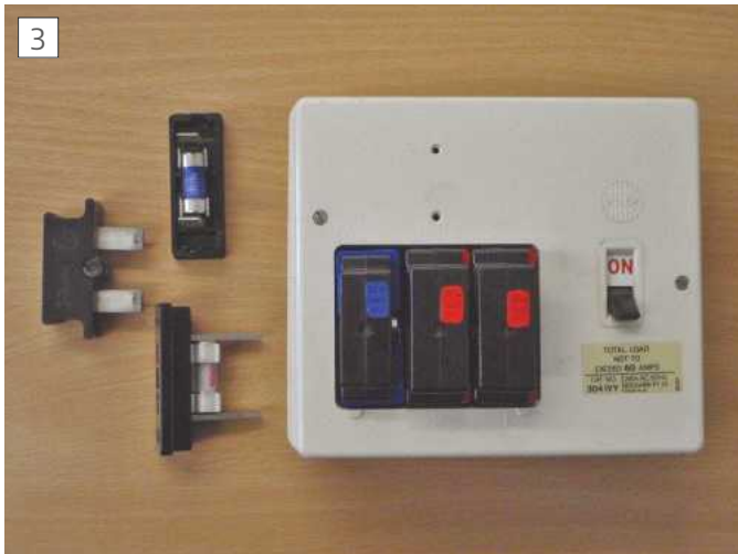
Distribution board with cartridge fuses.
