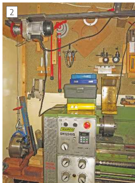
Winch installed above lathe.
