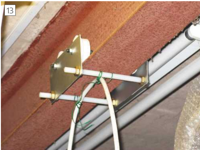
Cable trolley in position on RSJ
