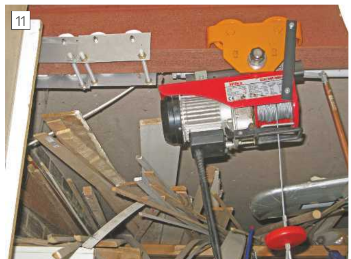
Hoist and trolley in position and showing bracket not working
