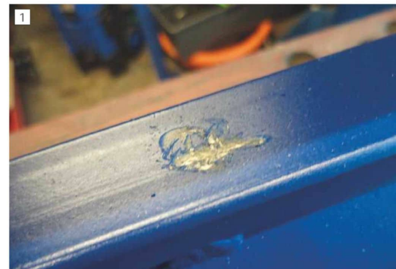
Witness mark showing the bolts had slipped.
