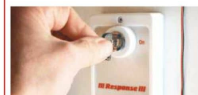
6 Use the key to activate alarm. This gives you, typically, 15 seconds to exit or enter your workshop
