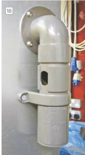
External view of dust extract duct showing the adjustable suction facility
