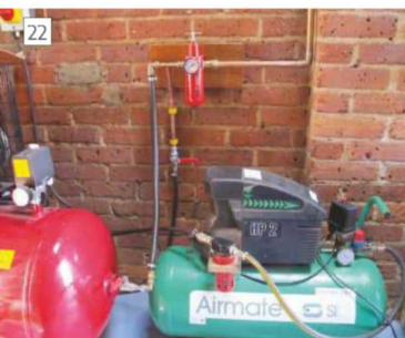
Light and heavy-duty compressors linked into my air distribution pipework
