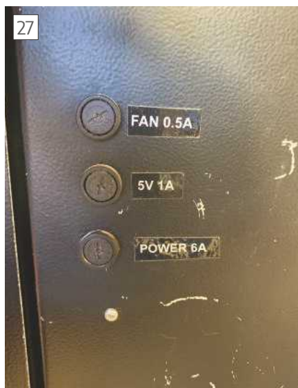
Fuses mounted mounted in the side of the cabinet.
