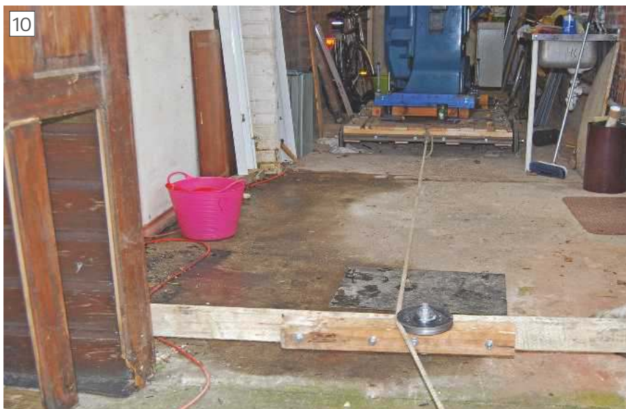
Guide Pulley at Rear of Garage
