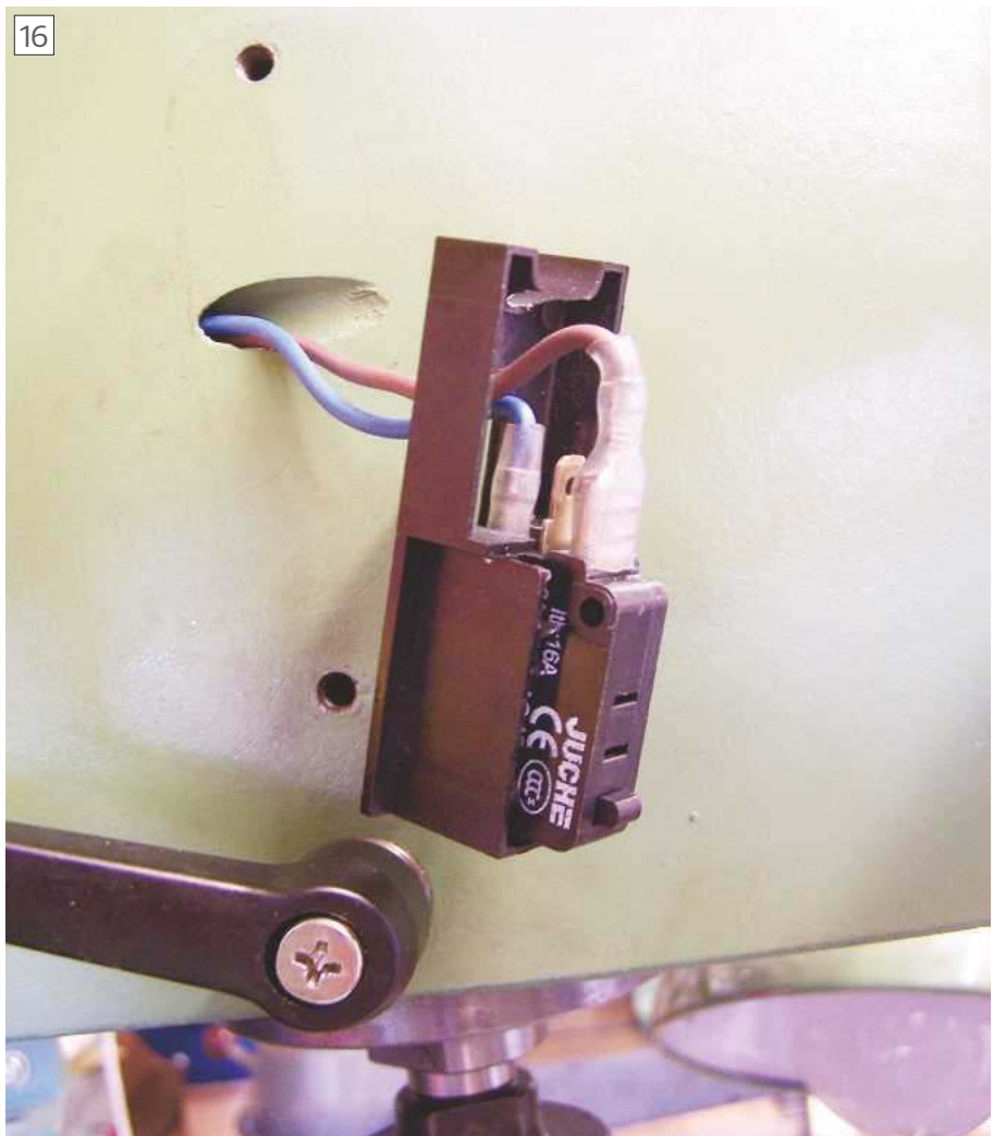
The guard interlock microswitch and existing cable.
