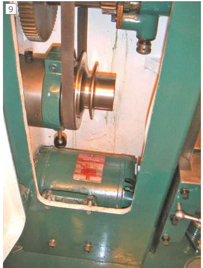
Looking down at motor
