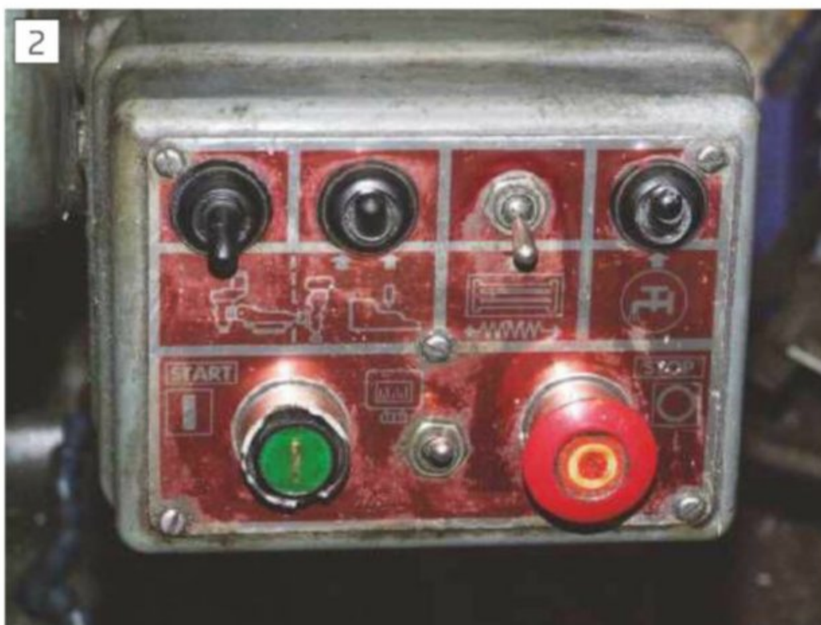
Operator Electrical Controls
