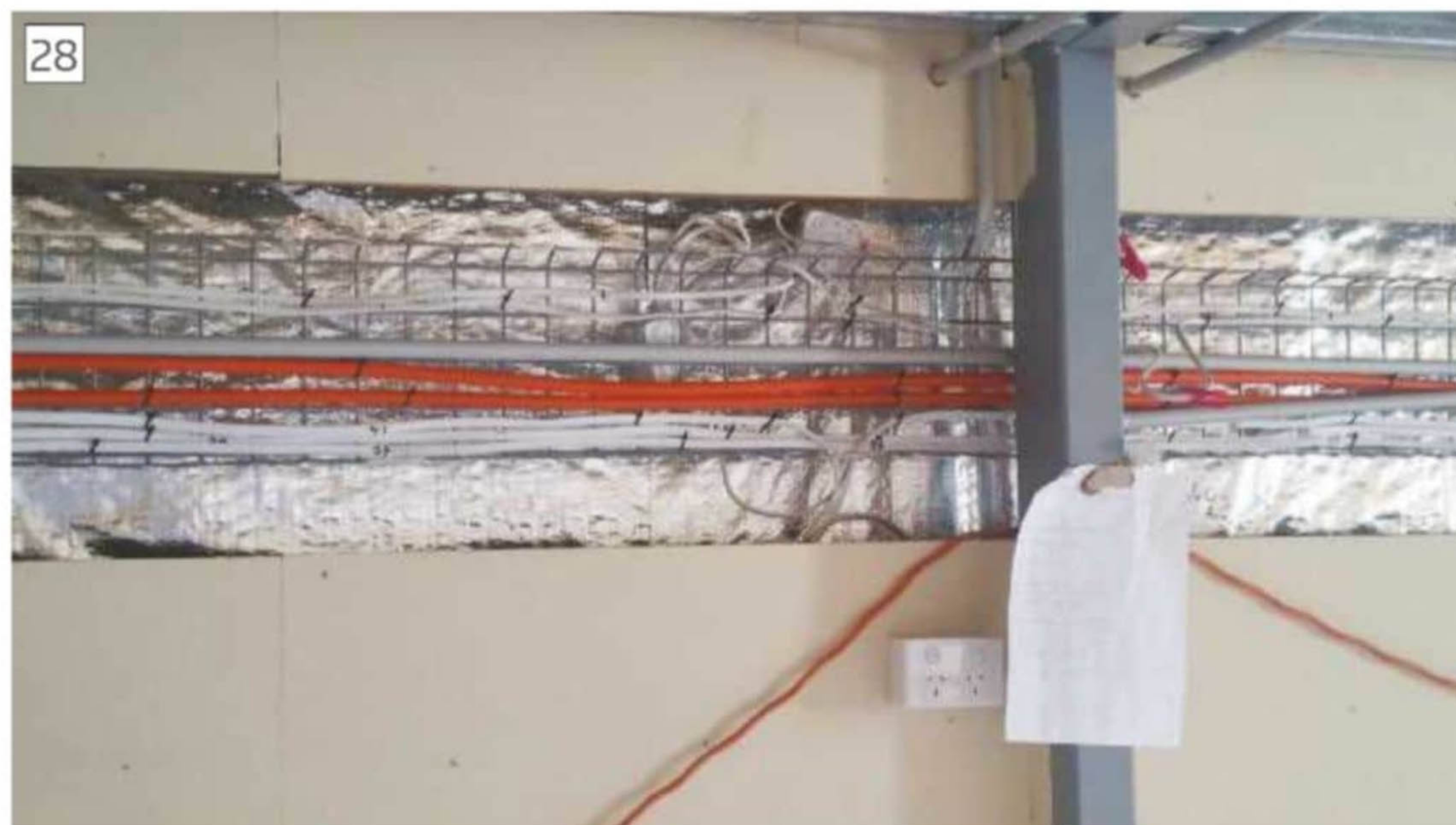
Cable ladder with cables in place
