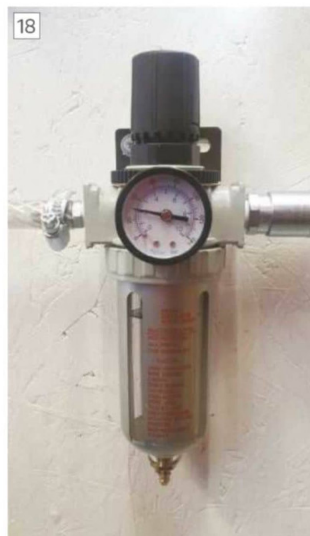
A wall mounted air regulator and moisture trap.
