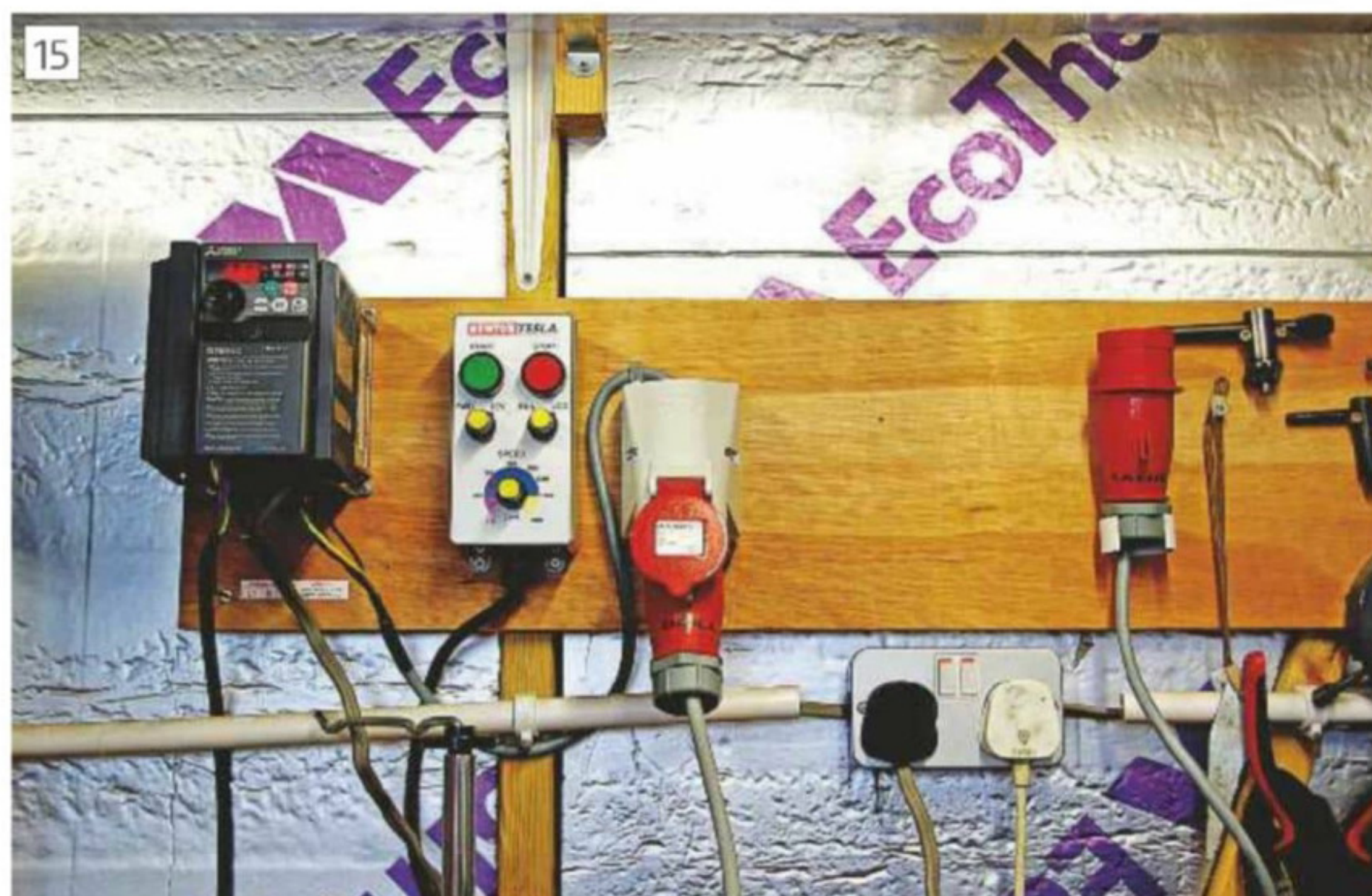
Three phase supply
