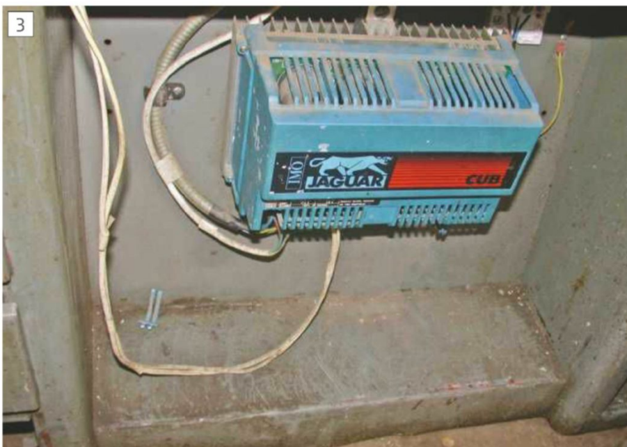
The original Jacobs Cub inverter. I tidied up that wiring as one of the first jobs!
