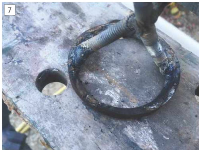
Equally noxious welding of the studding – but it held!
