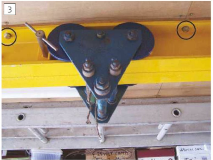
The trolley at the stop – between two of the mounting screws (circled)
