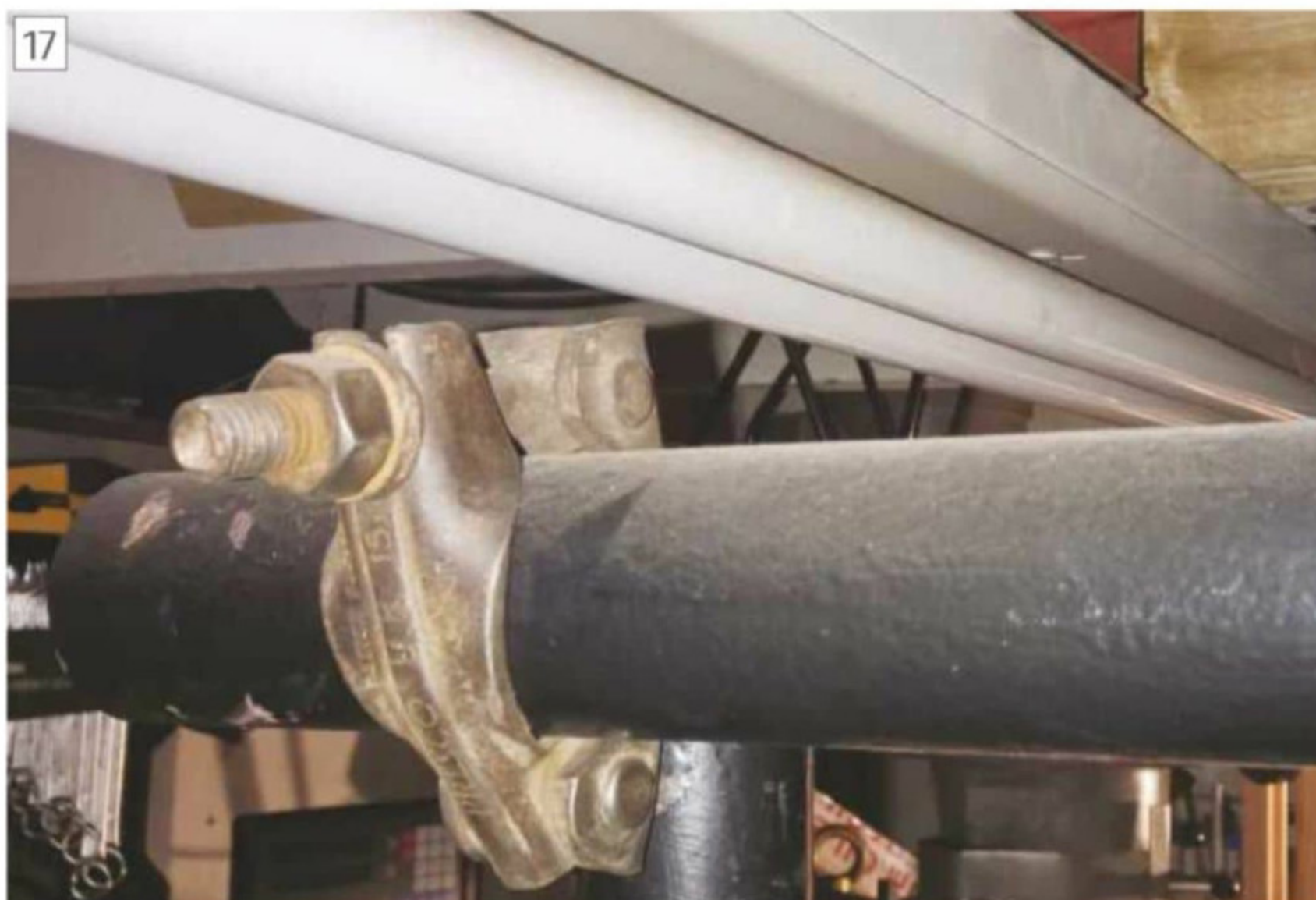
Just missing the fluorescent tube
