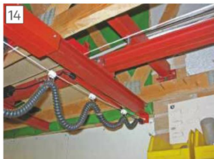
Power cable arrangement
